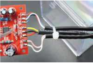
Arrange the wires neatly and fasten the wires with nylon cable ties.
